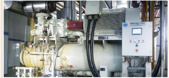
Air compressor at refrigeration plant
